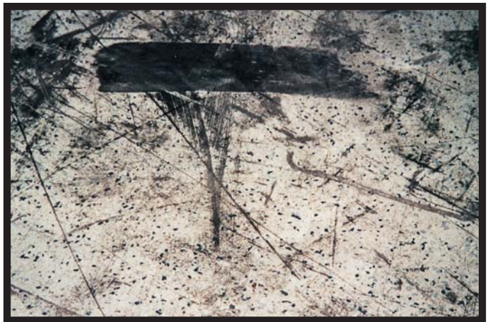
3. Although heavily soiled, the resilient vinyl tile has held up well under continuous forklift traffic.
