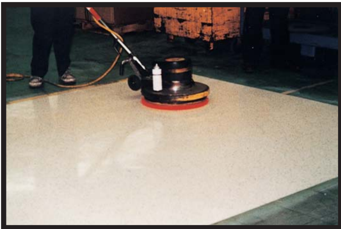
5. The clean floor was then polished with a low-speed buffer. The badly abused floor looks like new and NO WAX OF ANY KIND WAS USED.
